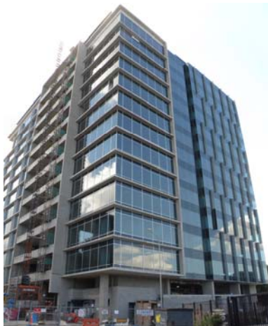
Green Square North Tower, Fortitude Valley on track for completion mid 2008 is presently 92% pre-committed (for details see page 4)
